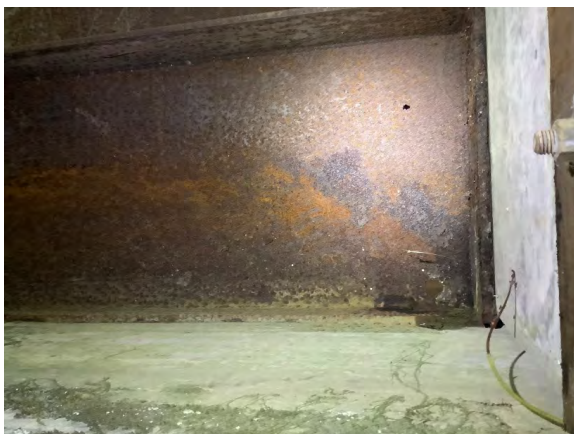
Upstream Profile - right side; rust scale
